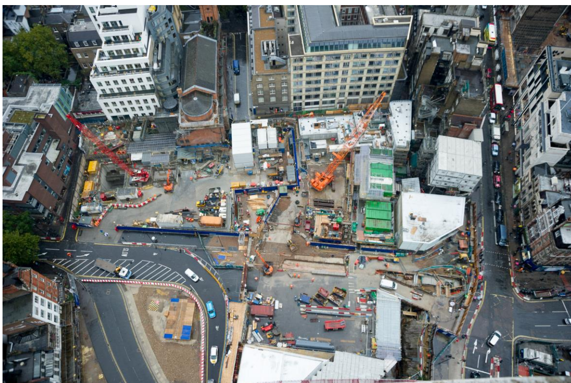
Current aerial view of the Tottenham Court Road Station Upgrade Project site
